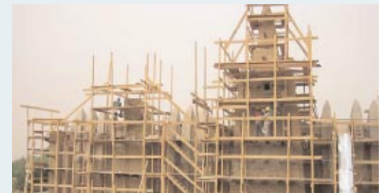
The completed scaffolding system along the east façade and central minaret. A chute, visible to the right of the minaret, was installed to facilitate the removal of debris from the roof of the mosque.
